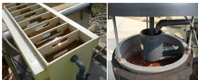
Fig. 4. Baffle weir used during the field trial (left) and close up photograph of effluent inlet and roughing filter at the feed-head, rotating filter head, and pelletised filter media in the filter column (right).
